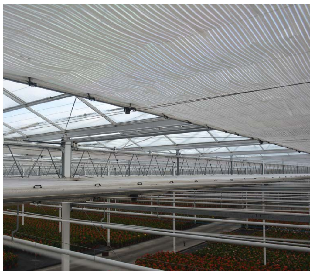
There is an energy screen and a shading screen in the greenhouse.
